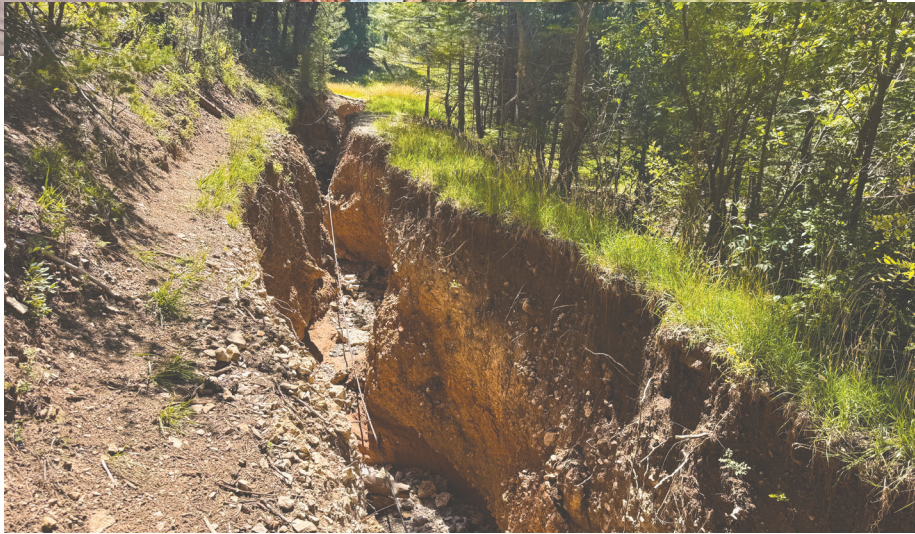
The washout below Toboggan Canyon, where the utility road used to be. Erosion has blocked large-equipment access to the 69kV line since 2018.
